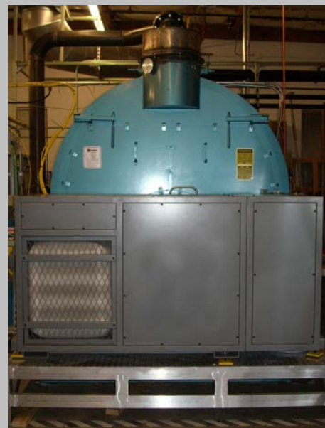
Combined heat and power system that meets boiler's thermal needs with added 100 kWe
